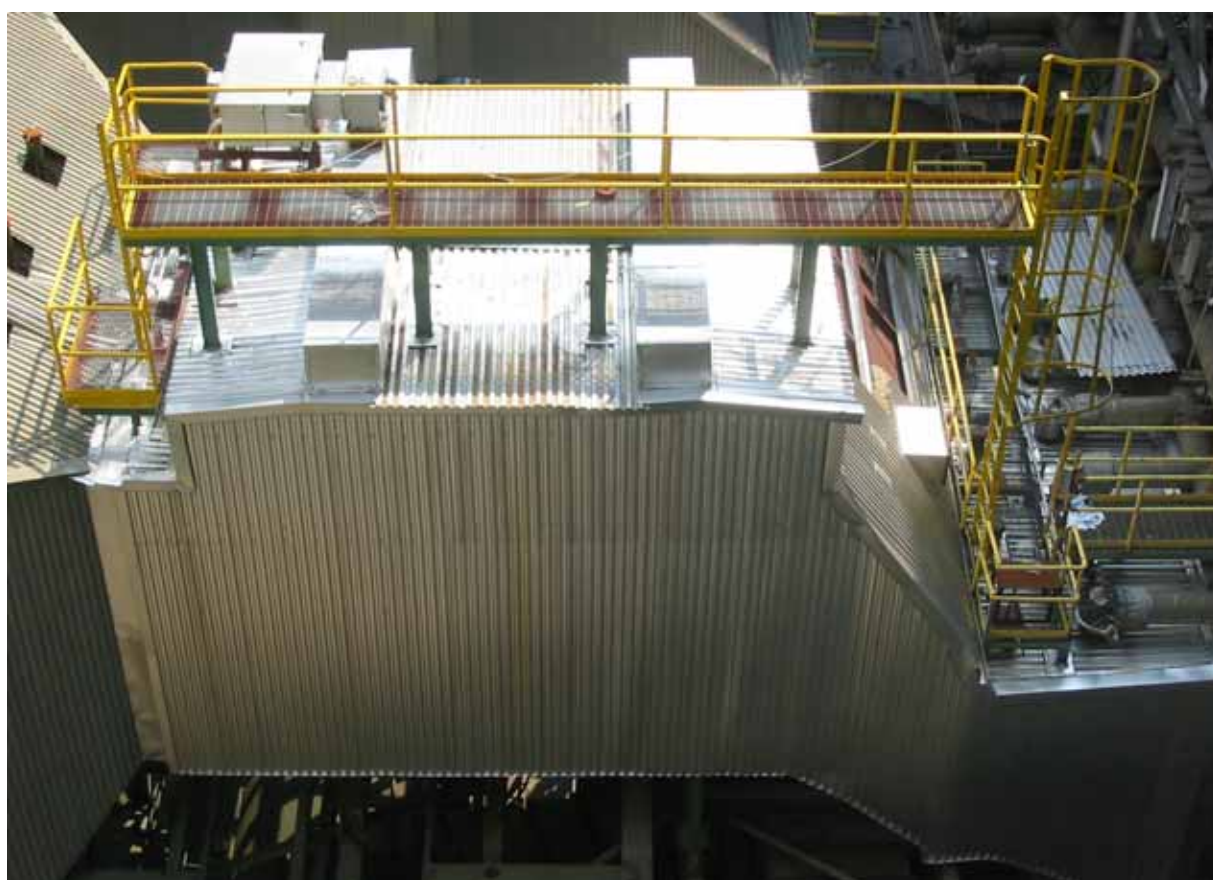
Photo 1. The Indigo Agglomerator installation at the Watson Plant.
